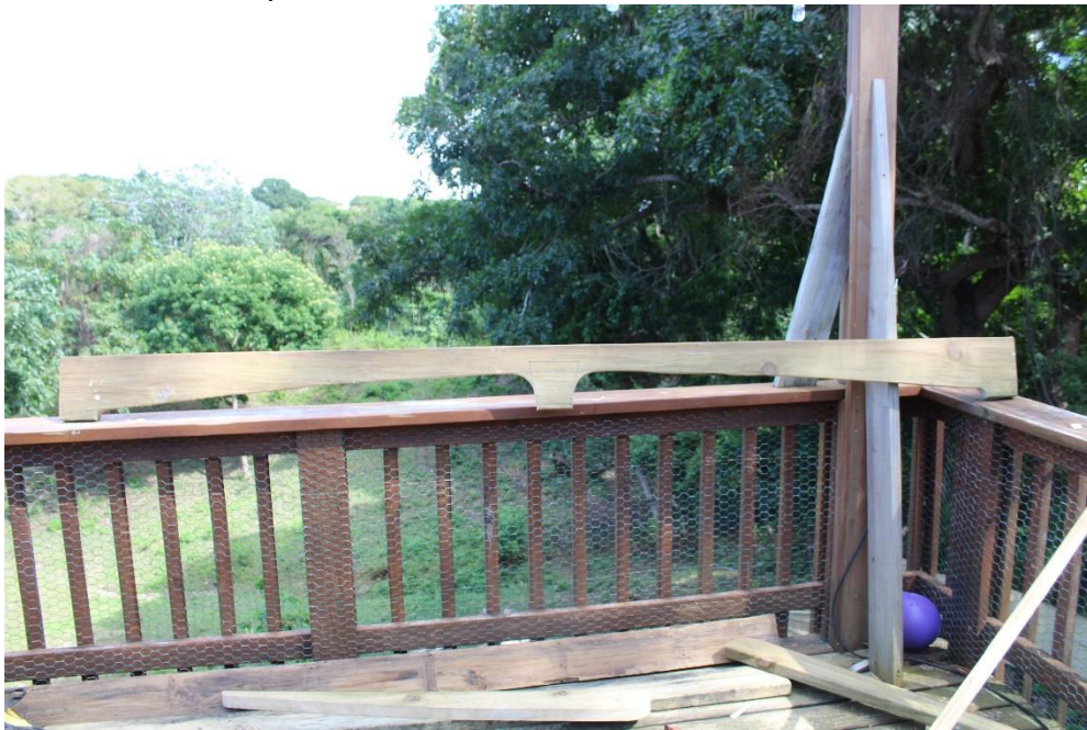
A jigsaw was then used to cut the arch and keystone profile.
